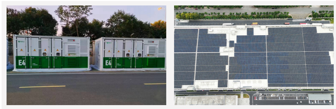
▲ Longshan Base II Power Storage Facilities
